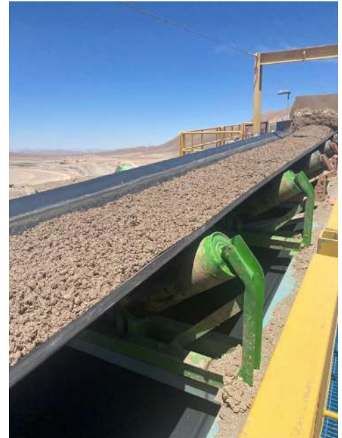
The installation of an ABG belt in one of the largest copper mining companies in Chile
